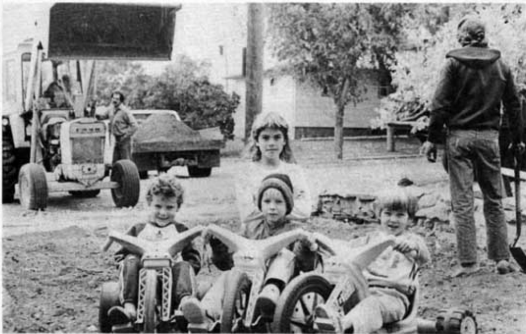
"How can we push the walls out to give us more living space?" Donavin and Cindy Grenz's solution in Linton, N.D.: build a garage with a bedroom on top. So Donavin Grenz (background, right), David Grenz (backhoe operator), and "Country," leaning on his shovel, set to work, preparing for the foundation. The kids even help with their three-wheeler entertainment for the grownups! Left to right: Justin Grenz, Jack Dockter (son of Dean and Judy Dockter), Eric Grenz, and Tana Grenz (back row).
