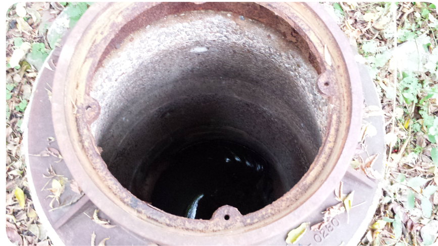
Figure 3.14: An severe example of the existing conditions of the sewer system (missing cover, not repaired) along Cascade Creek. (Photo Credit: Josh Wildt, October 2013)
