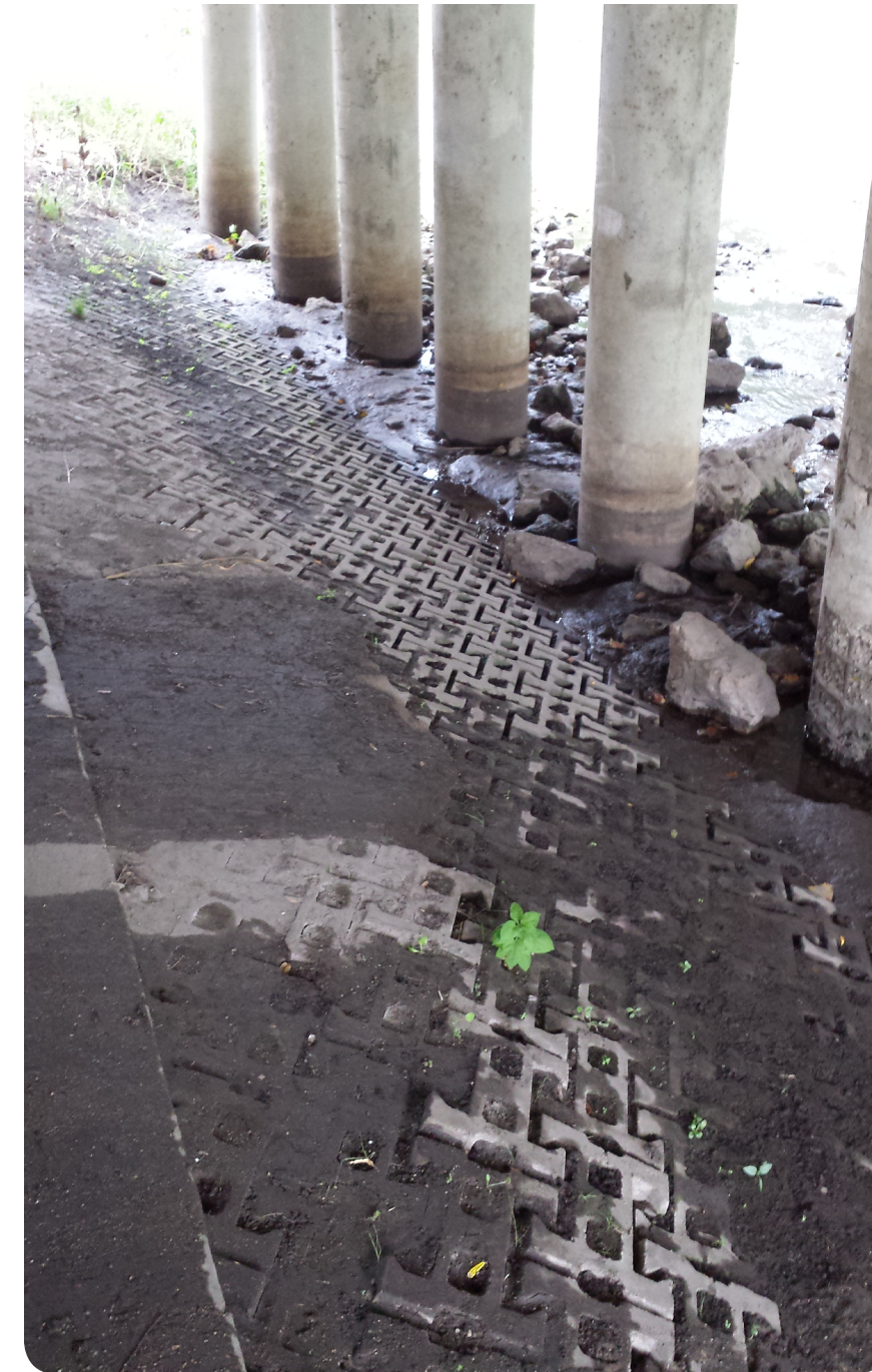
Figure 3.8: Concrete riprap found along Cascade Creek (Photo Credit: Josh Wildt)
