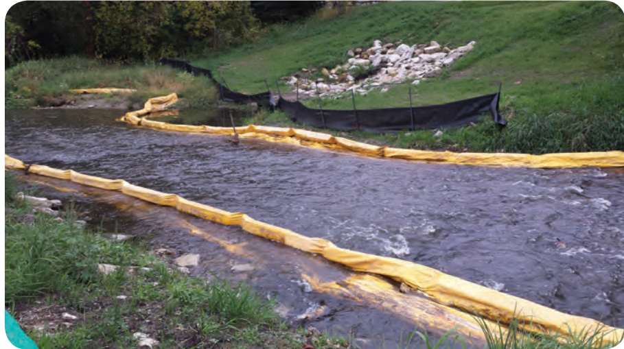
Above: Temporary relief from erosion problems.
