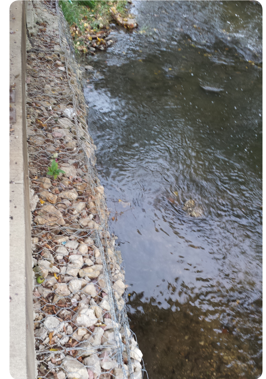
Figure 3.: Recycled concrete in wire baskets used for erosion control along Cascade Creek. (Photo Credit: Josh Wildt, October 2013)
