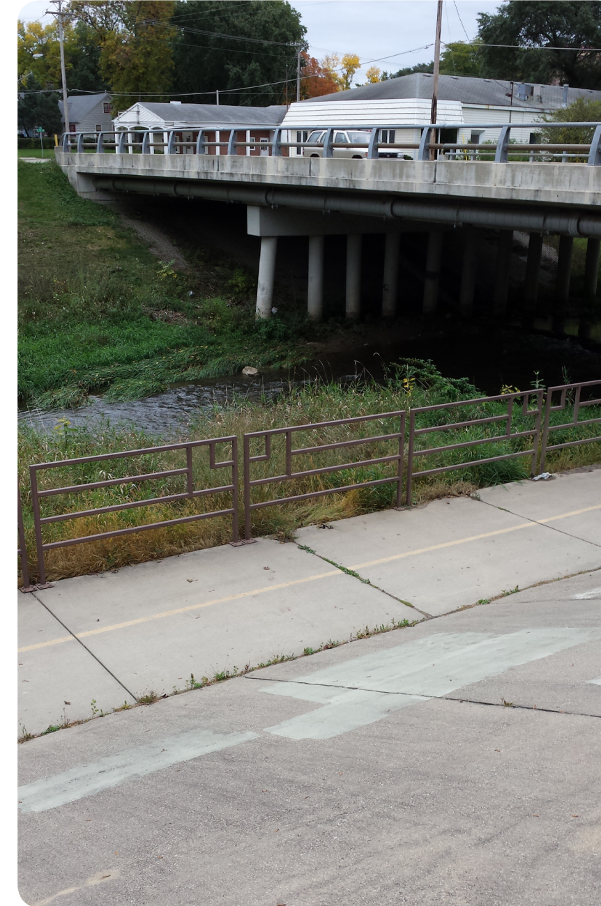
Figure 3.: Concrete creek banks located in some of the most channelized portion of Cascade Creek. (Photo Credit: Josh Wildt, October 2013)
