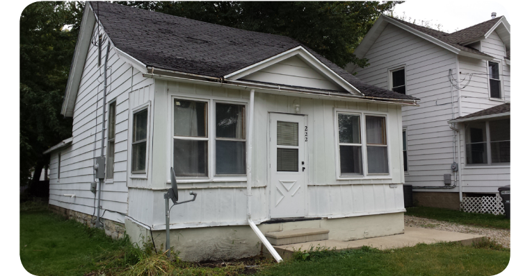
Figure 3.2: House in need of repair in Kutzky Neighborhood (Photo Credit: Josh Wildt)
