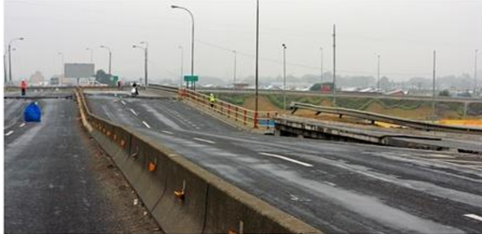
Fig. 1.6. Liquefaction-induced settlement of pier foundations for Juan Pablo II bridge [4]
