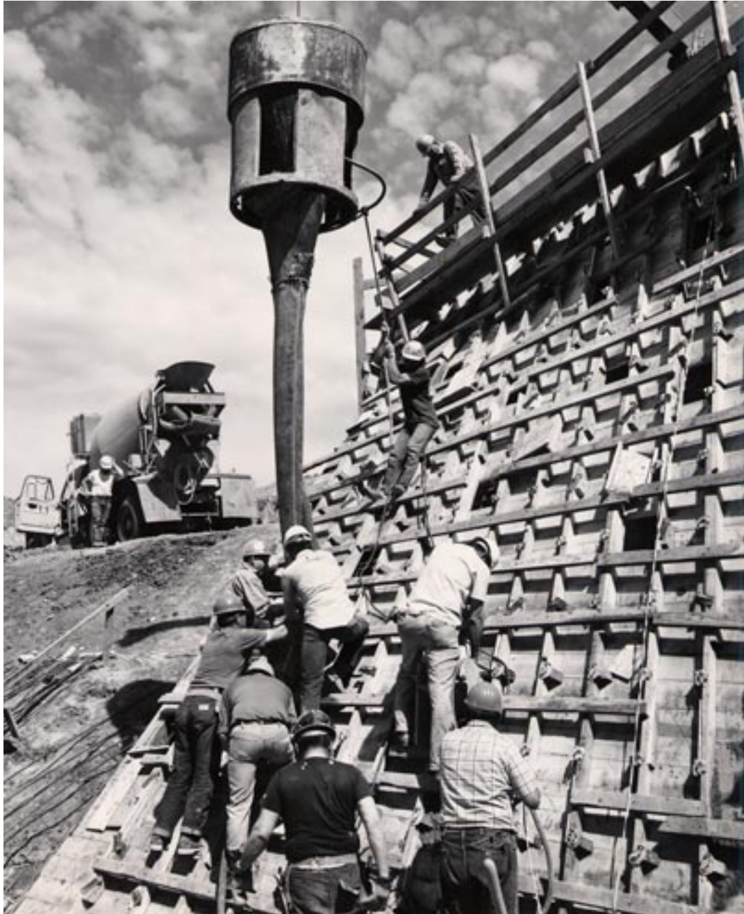
Concrete work on the McClusky Canal, ND, 1972. (Garrison Diversion Conservancy District, Bureau of Reclamation, Department of the Interior)
