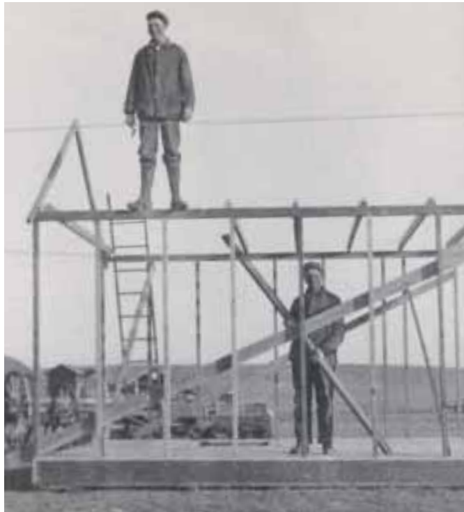
Raymond Pfundheller (brother) and Henry Pfundheller (father) of Nora, building her homestead shack, 1913. (Nora Pfundheller King, Lenartz)
