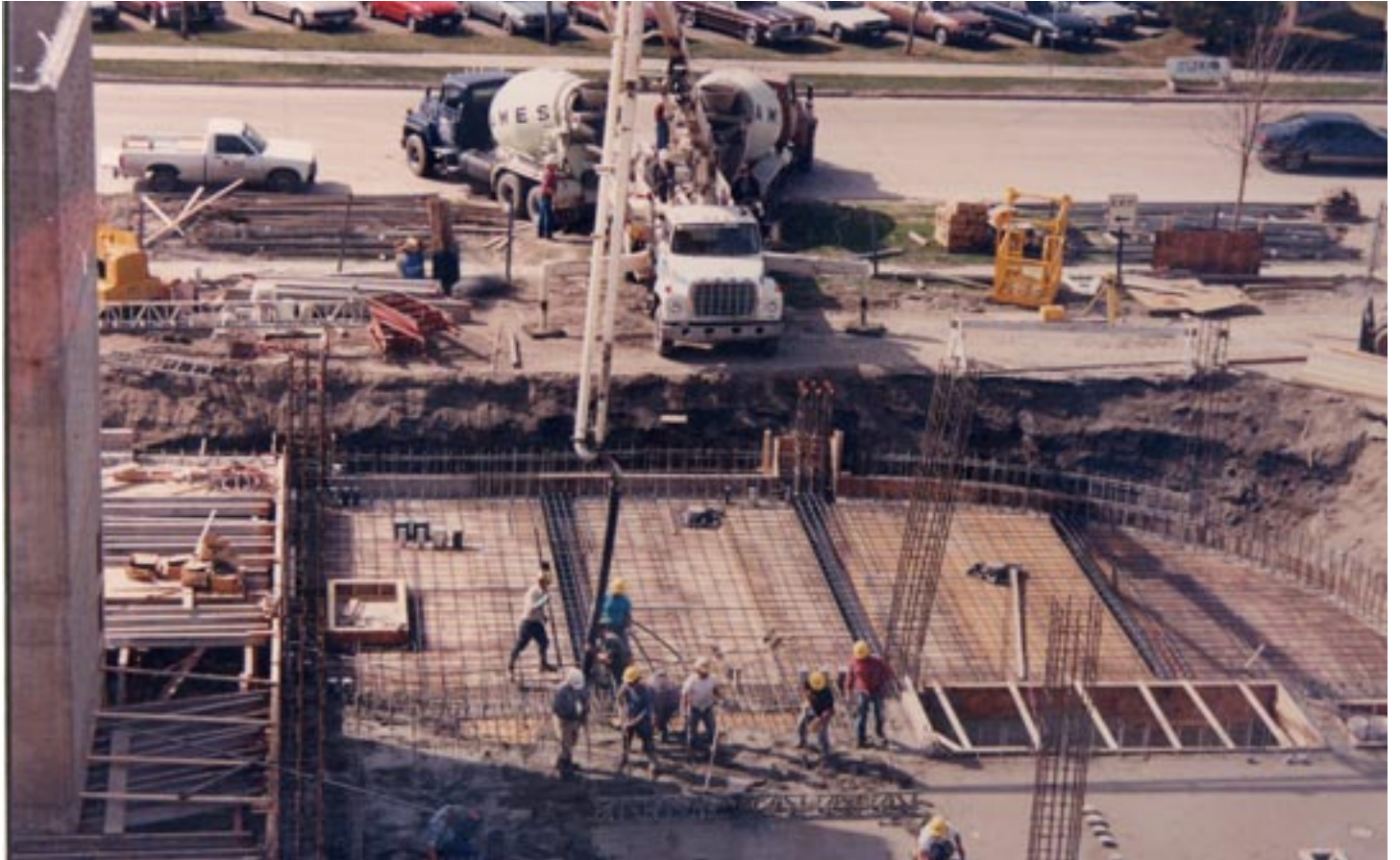
Constructing an addition to Dakota Hospital, Fargo, 1992. Meinecke-Johnson Company and Ames Sand & Gravel, 1992. (Ames Sand & Gravel)
