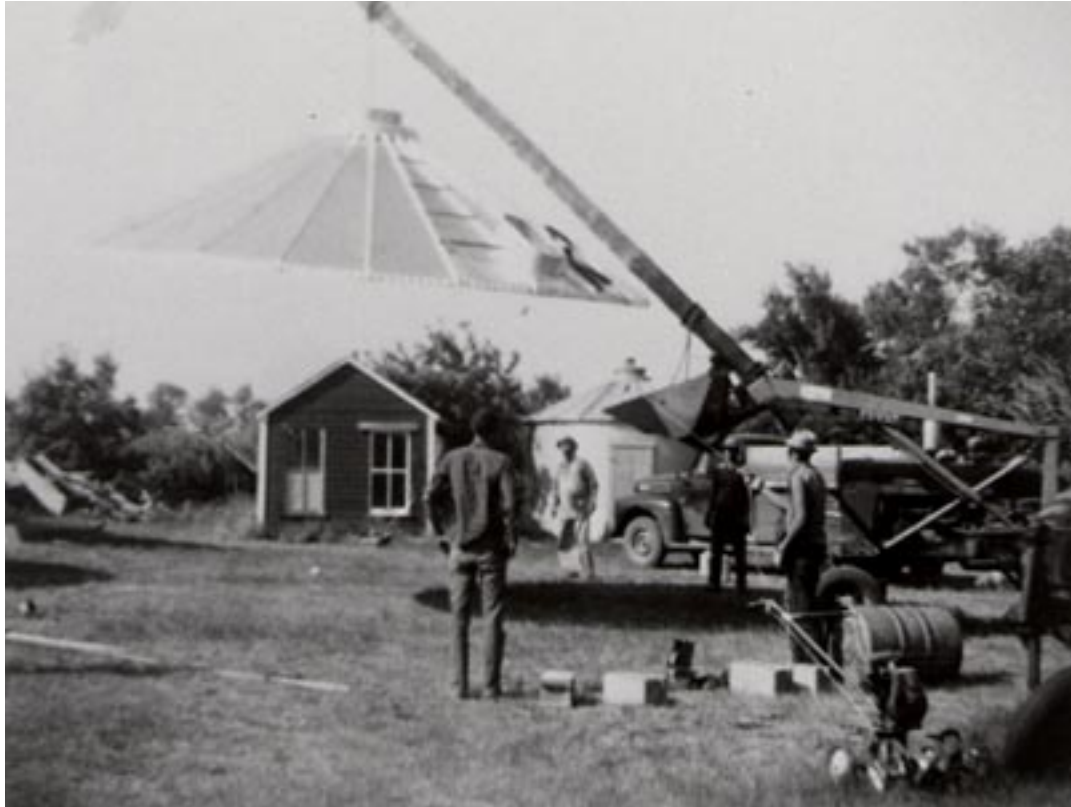
Raising the roof to a grain bin. Neighbors, Stan Swanson, Hank Wirty, Shorty Wirty, Harley Hassler, and Tracy Scott gathered to help Grandpa Jake Hepper, and his son Russell. "Very hot. Hoisted the roof on in the afternoon. The pole slipped and dropped the roof to the ground. Almost overturned the tractor." (Personal journal, July 23, 1963.)
