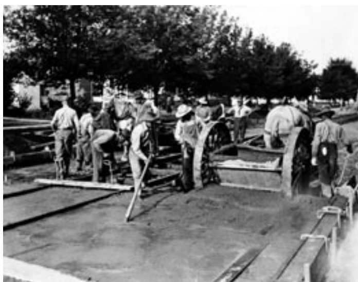
Laying concrete on either side and between street car rails in Moorhead, MN, 1920s. (IRS, NDSU, Fargo, 2063.29.29)
