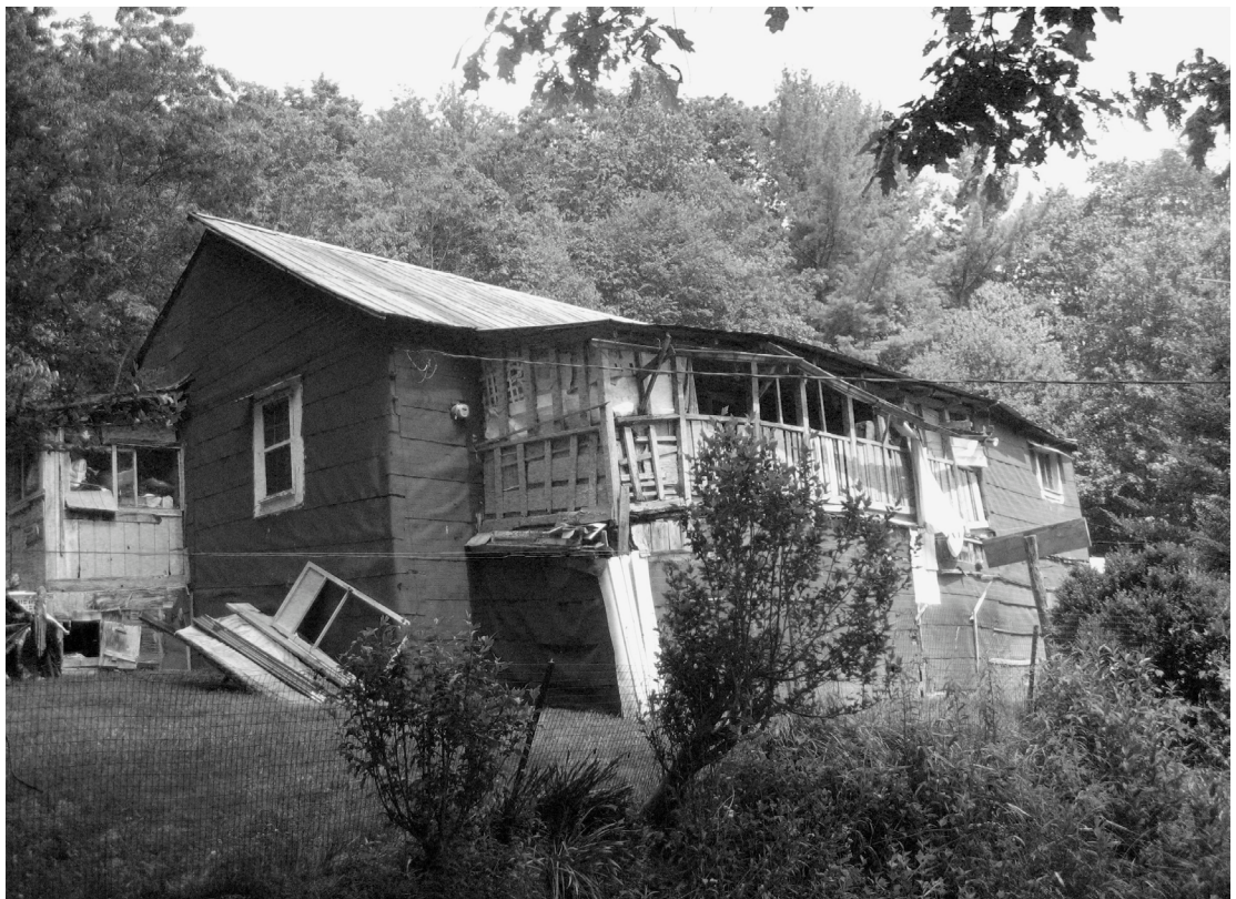
Fig 2.1: A home near Mountain City, TN before ASP volunteers and staff began repairs.
