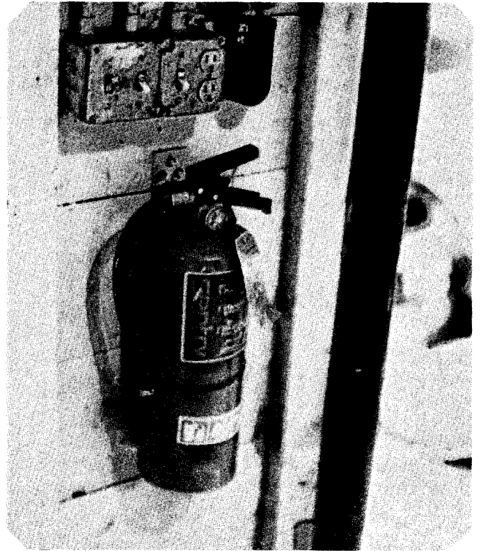
Fire extinguishers mounted in buildings should be easy to find and easy to reach.
