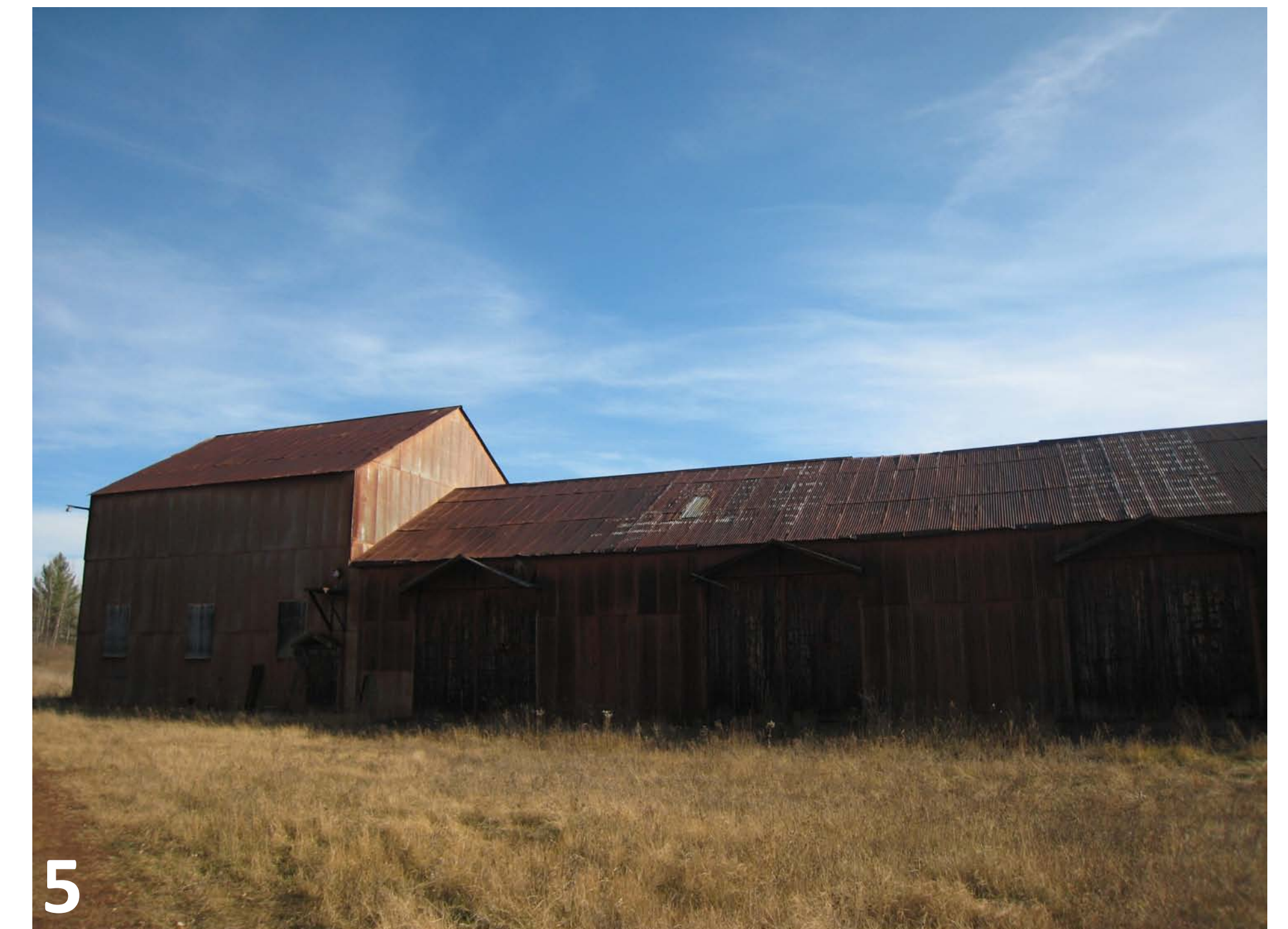
Former Sintering Warehouse -in disrepair -full of debris/garbage -a lot of character
