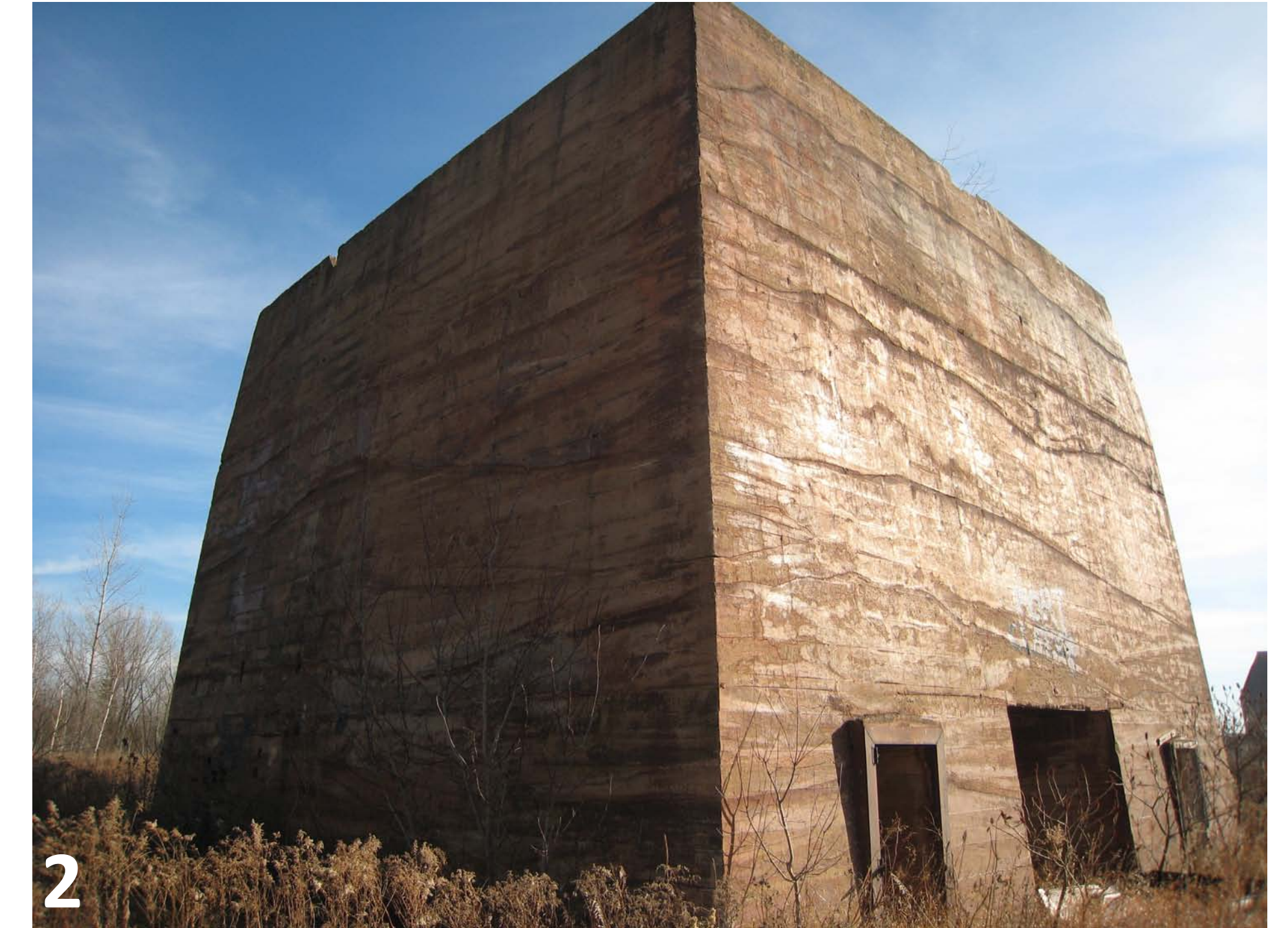
Former Sintering Furnace -overgrown -in need of minor repair -a lot of character
