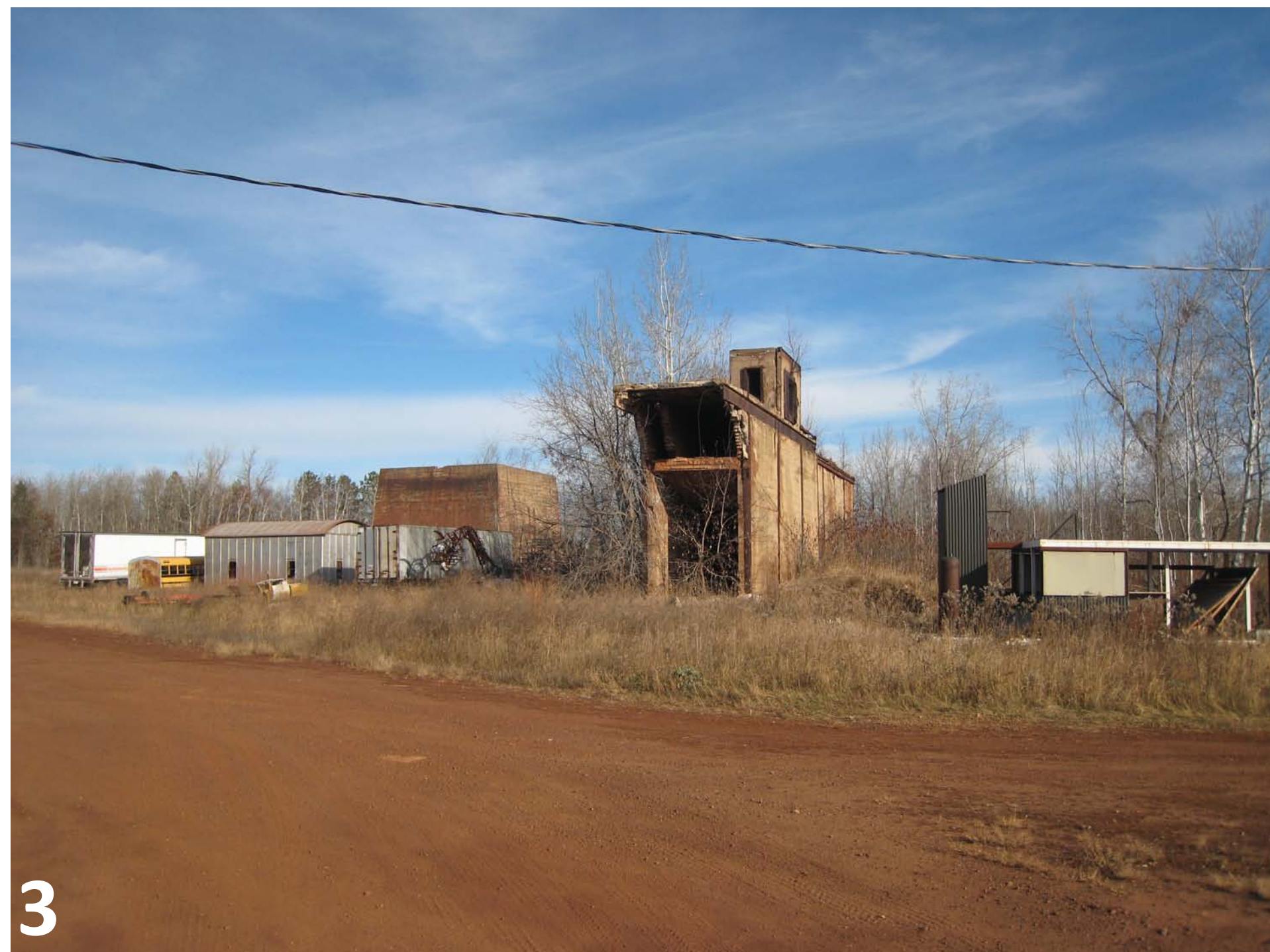
Former Sintering Elevator -in disrepair -overgrown -a lot of character
