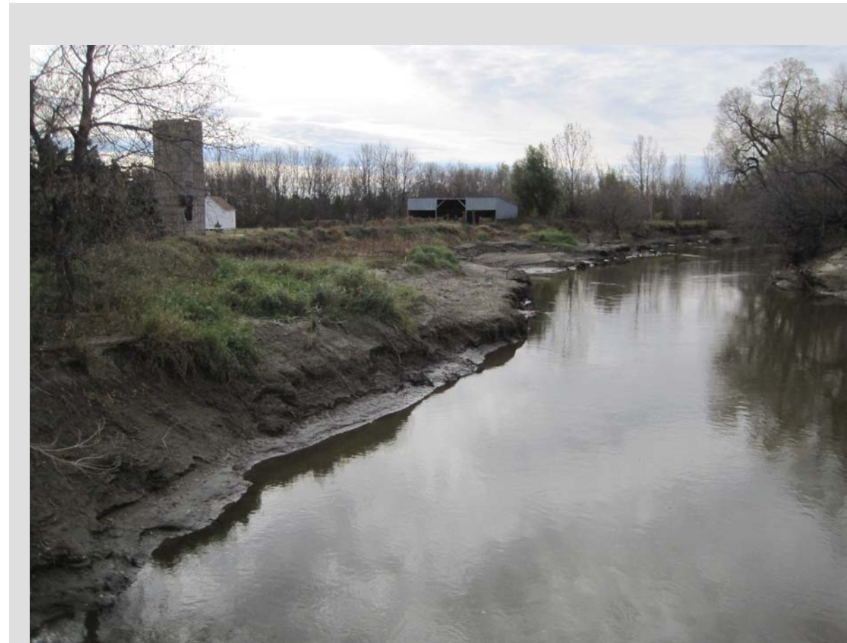
Figure 8. Erosion of the Sheyenne River in Horace, North Dakota. (Source: Candice D’Arcangeli)
