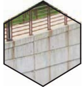
concrete retaining wall & rusted metal railing
