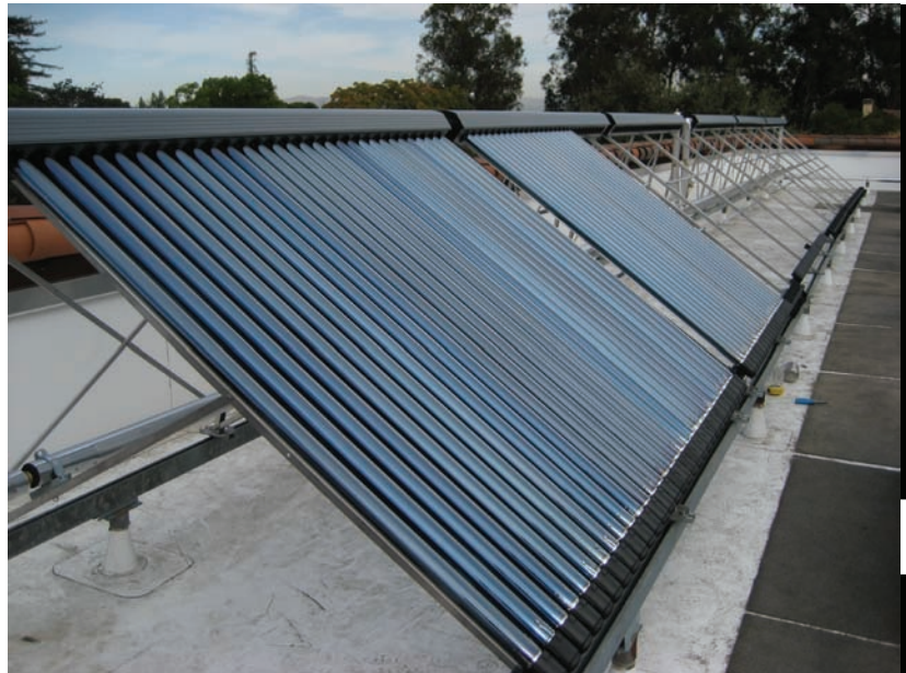
Solar water heaters
