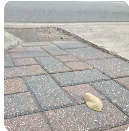
Figure 1.12: Pavers are sinking next to concrete sidewalk.
