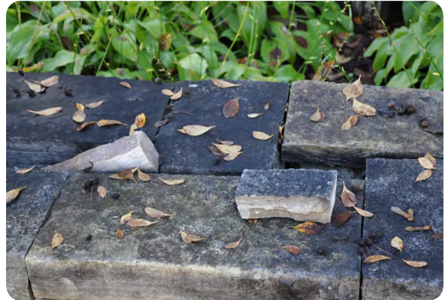
Figure 5.1: Deteriorating feature that will be redesigned to create a longer life expectancy.
