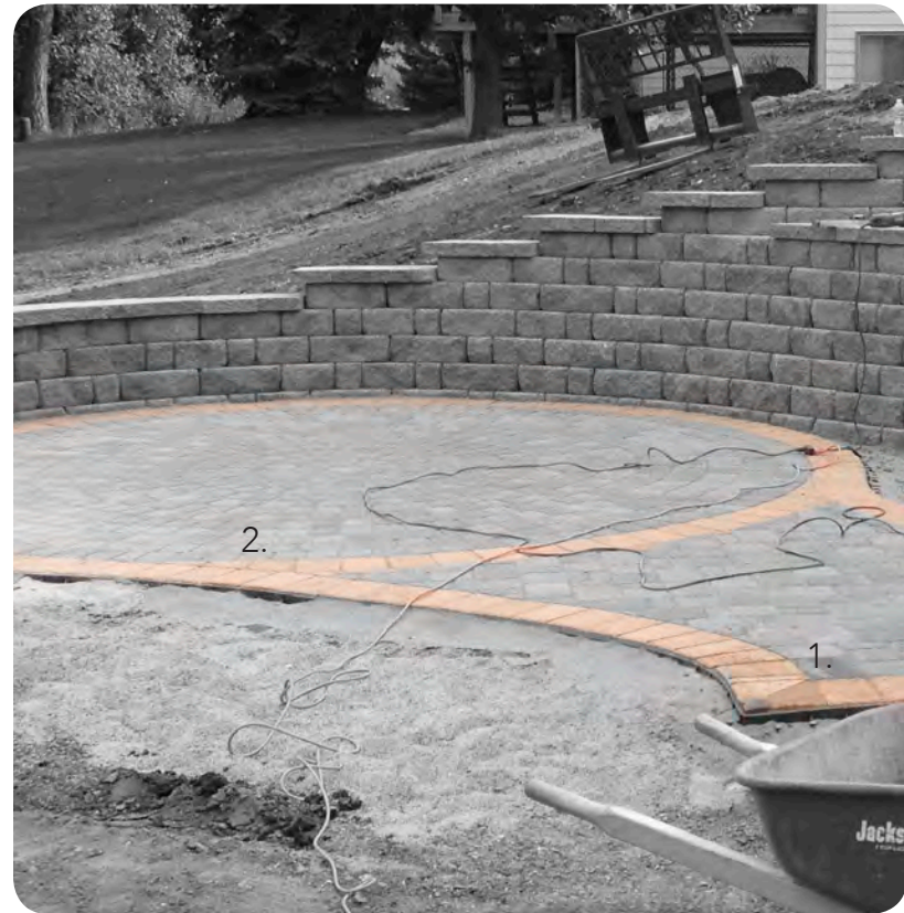
Figure 1.1: The soldier course on this patio was built with craftsmanship. The 90 degree corner was miter cut (1), and the soldier course around the circle was tied into the boarder soldier course (2).
