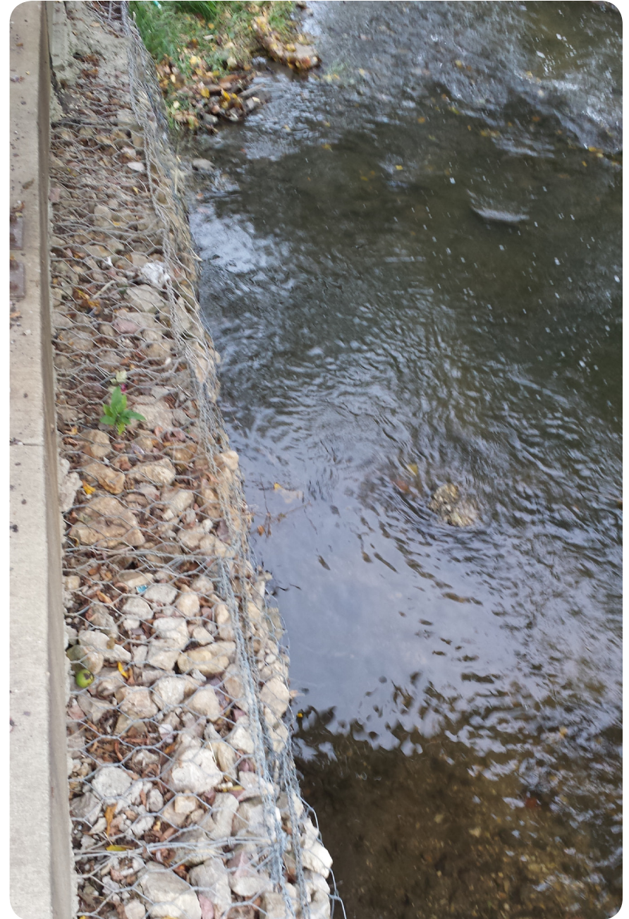
Figure 3.: Recycled concrete in wire baskets used for erosion control along Cascade Creek. (Photo Credit: Josh Wildt, October 2013)
