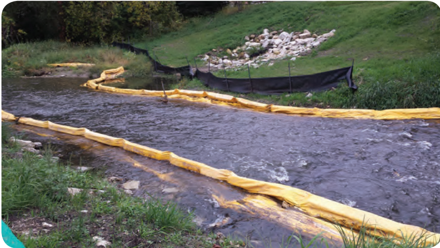
Above: Temporary relief from erosion problems.
