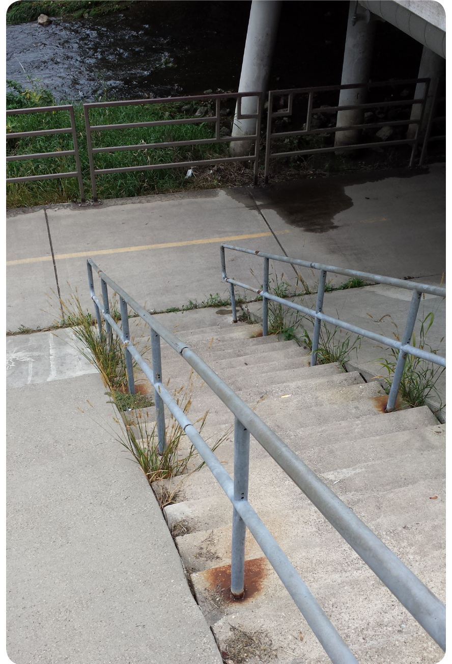
Figure 3.: Stairs built into concrete banks to allow human access. (Photo Credit: Josh Wildt, October 2013)
