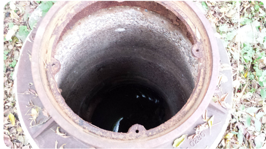
Figure 3.14: An severe example of the existing conditions of the sewer system (missing cover, not repaired) along Cascade Creek. (Photo Credit: Josh Wildt, October 2013)
