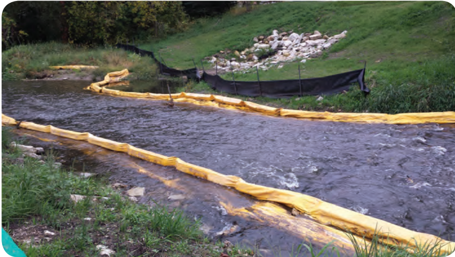
Above: Temporary relief from erosion problems.
