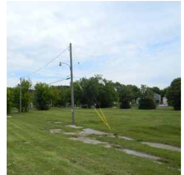
figure 24.1: above ground utilities
