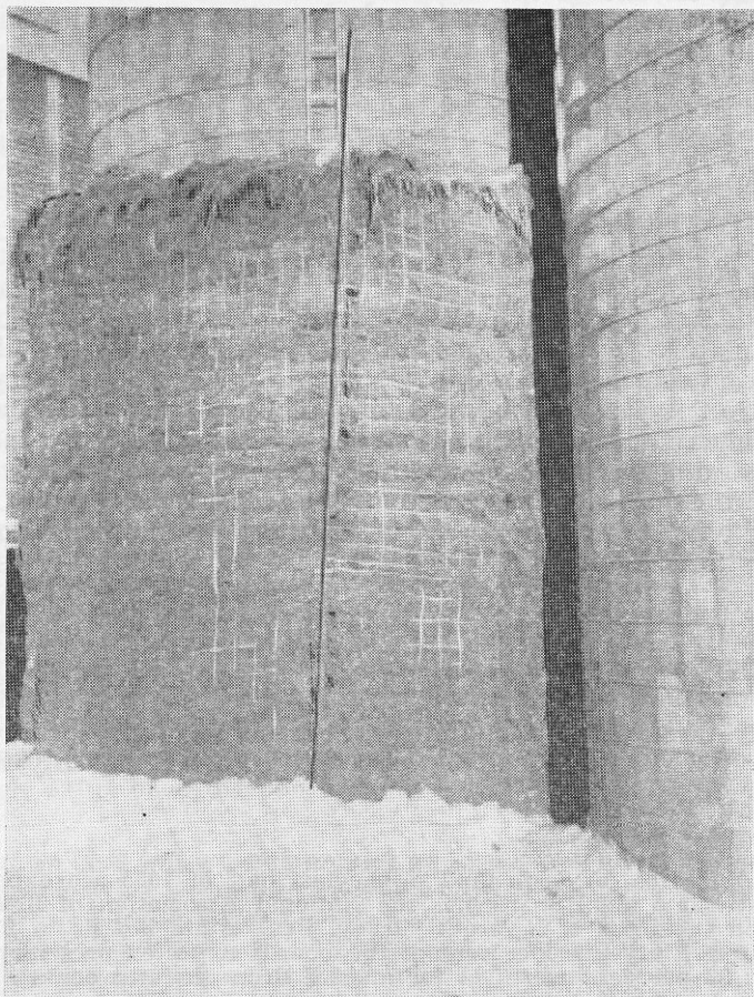
FIGURE 3.—Flax straw insulation in place around the lower 14 feet of the upright concrete stave silo.
