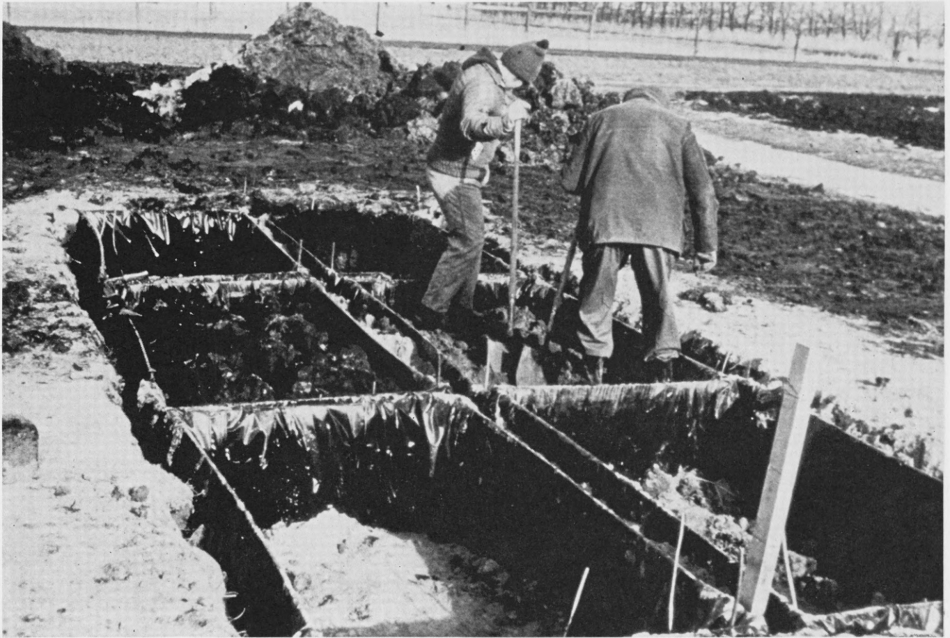
Figure 5. Filling and packing soil in the lysimeters after the drainage systems were installed.
