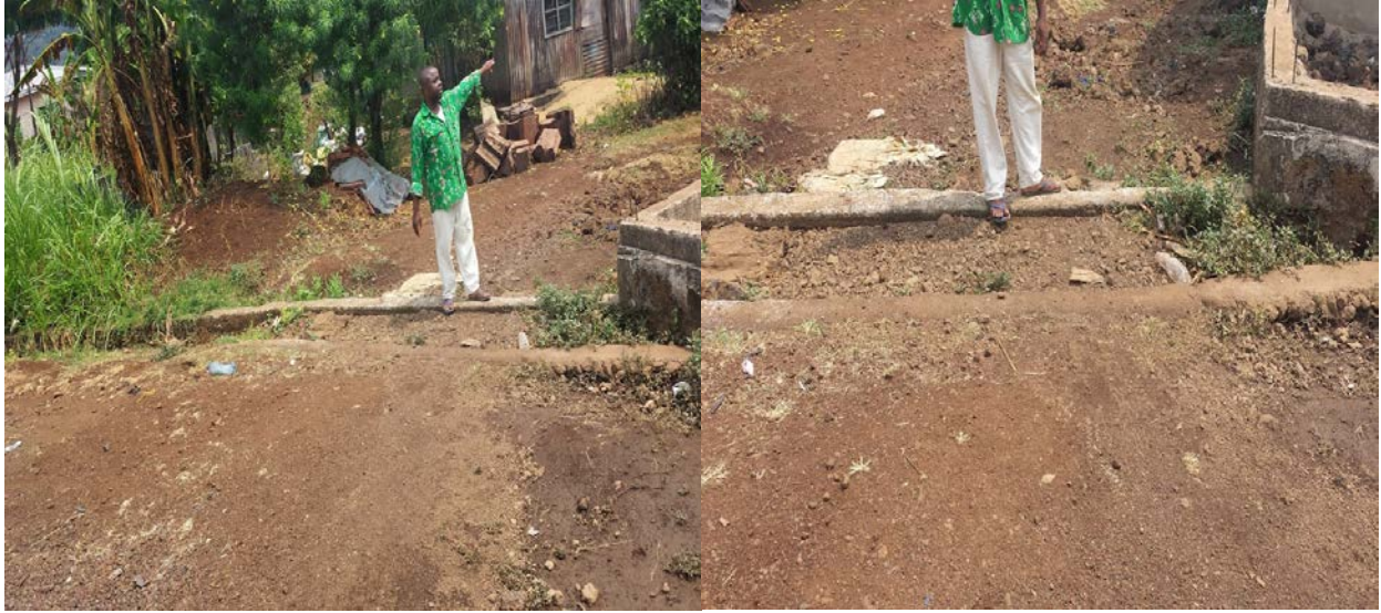
Figure 7. Blocked gutters in a village near Limbe
