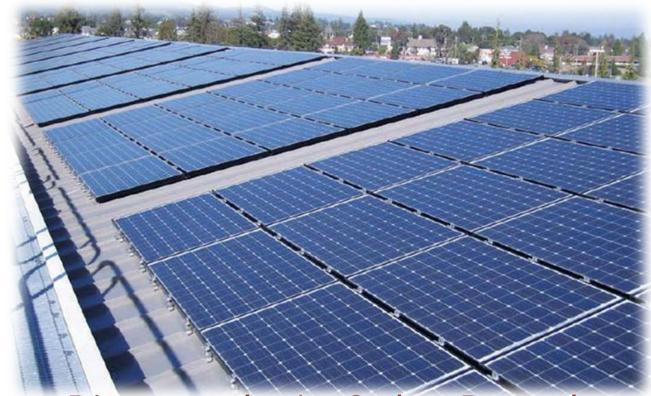
Photovoltaic Solar Panels
