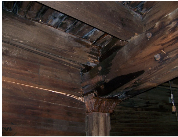
Water damaged beam
