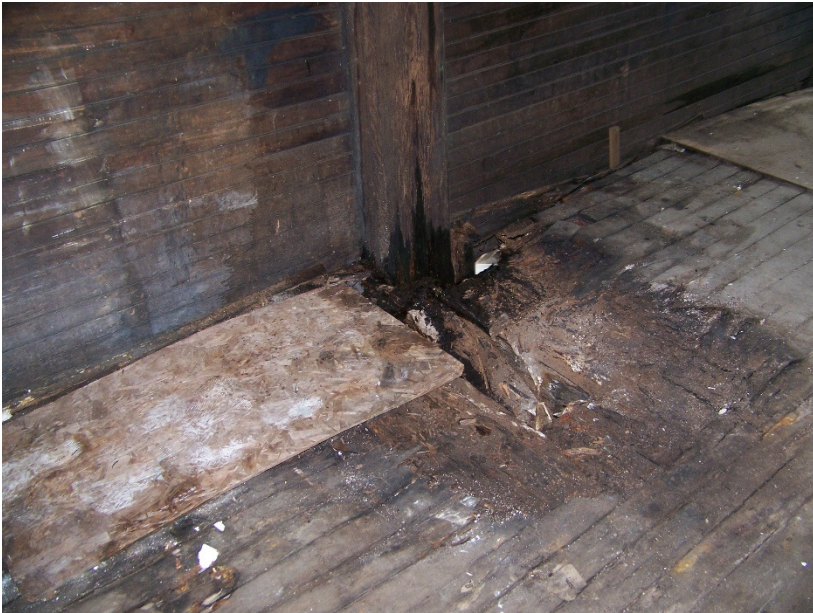
Water damaged floor
