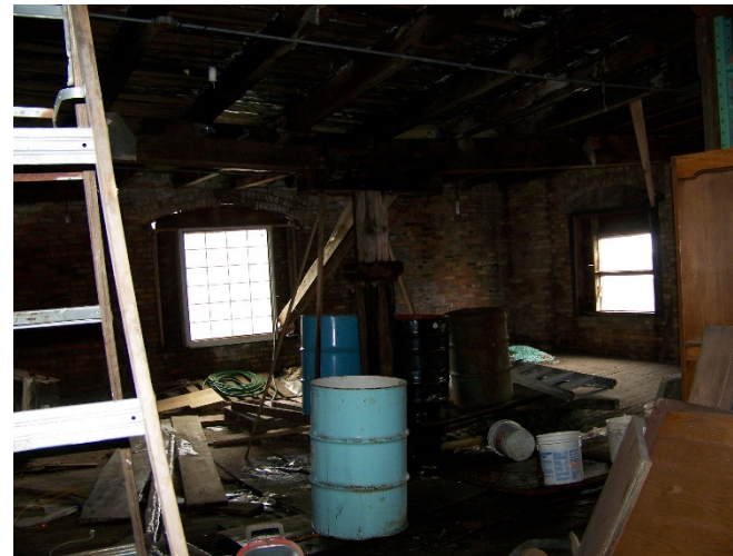
North East corner with most water damage
