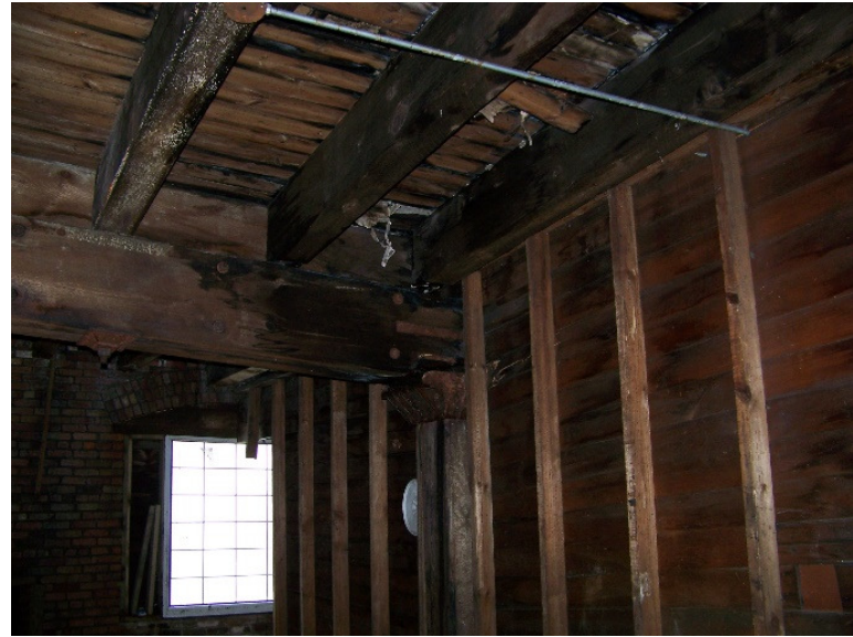
Water damaged structure
