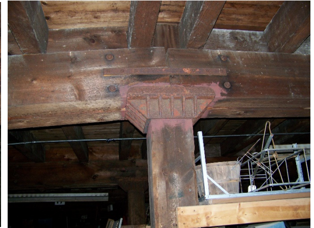
Result of sagging beam
