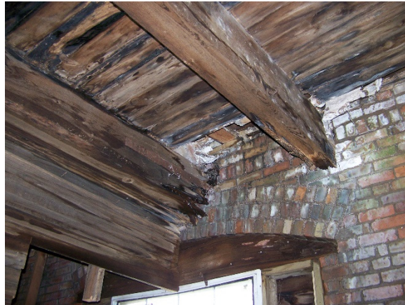
Result of water damage
