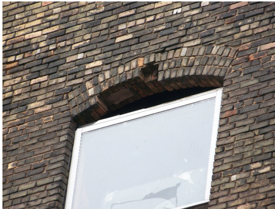
Damaged brick at window
