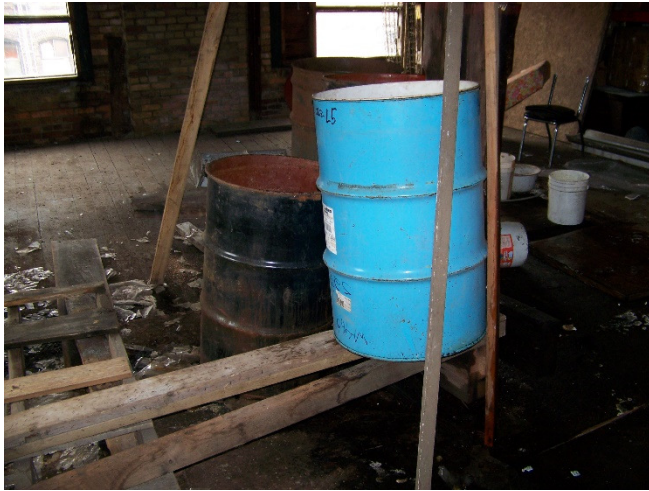
Water damaged top floor
