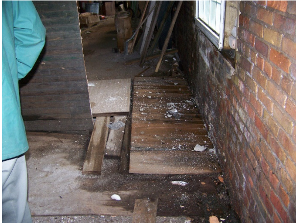
Water damaged floor
