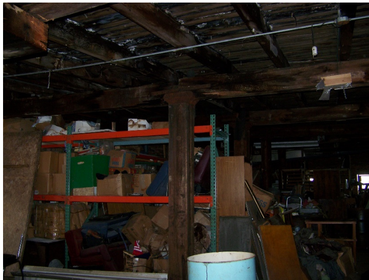
Underside of slightly water damaged floor
