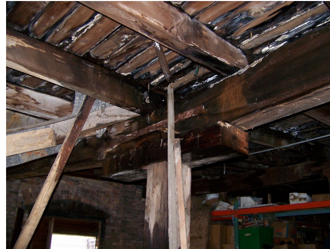
Underside of water damaged roof
