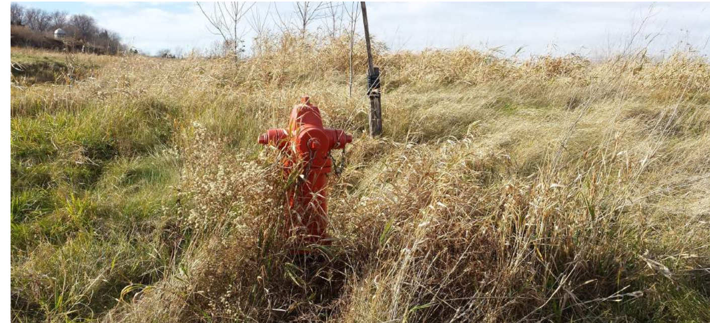
Figure 39 | Image of fire hydrant west of the site
