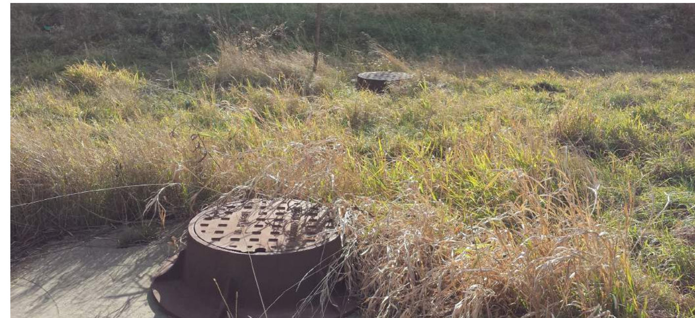
Figure 40 | Image of manhole covers for sewer access south of site
