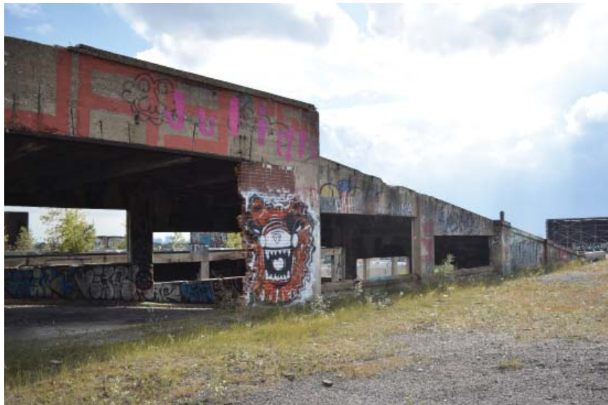
[67] A ramp at the end of the north building brought completed Packards to the street. Today it leads up to a prairie-like rooftop view of downtown Detroit.
