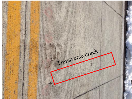
Figure 11. The occurrence of transverse cracks on adjacent panel of crack sensors (1D-4 & 1D-5).
