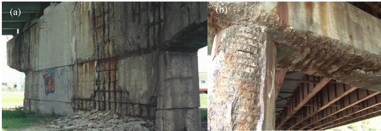
Figure 1-2. Typical corrosion-induced damages on (a) abutment and (b) pier (Gergely et al., 1998; Hansson, 1995)
