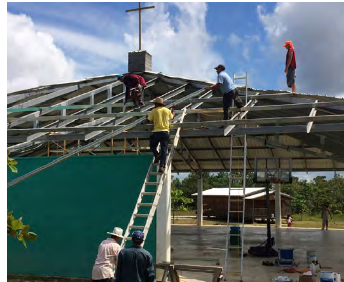
FIGURE 3: VOLUNTEERS FROM LOCAL CHURCH REPAIRING ROOF the local community in the building process (figure 3). However, that is not always the case and can certainly be improved on still in the case of the three teams I saw. Something detrimental that can happen with bringing in outside groups to do work is that the locals don’t actually get the valuable experience they could use. Furthermore, in the case of building a community building, if there were no locals engaged
