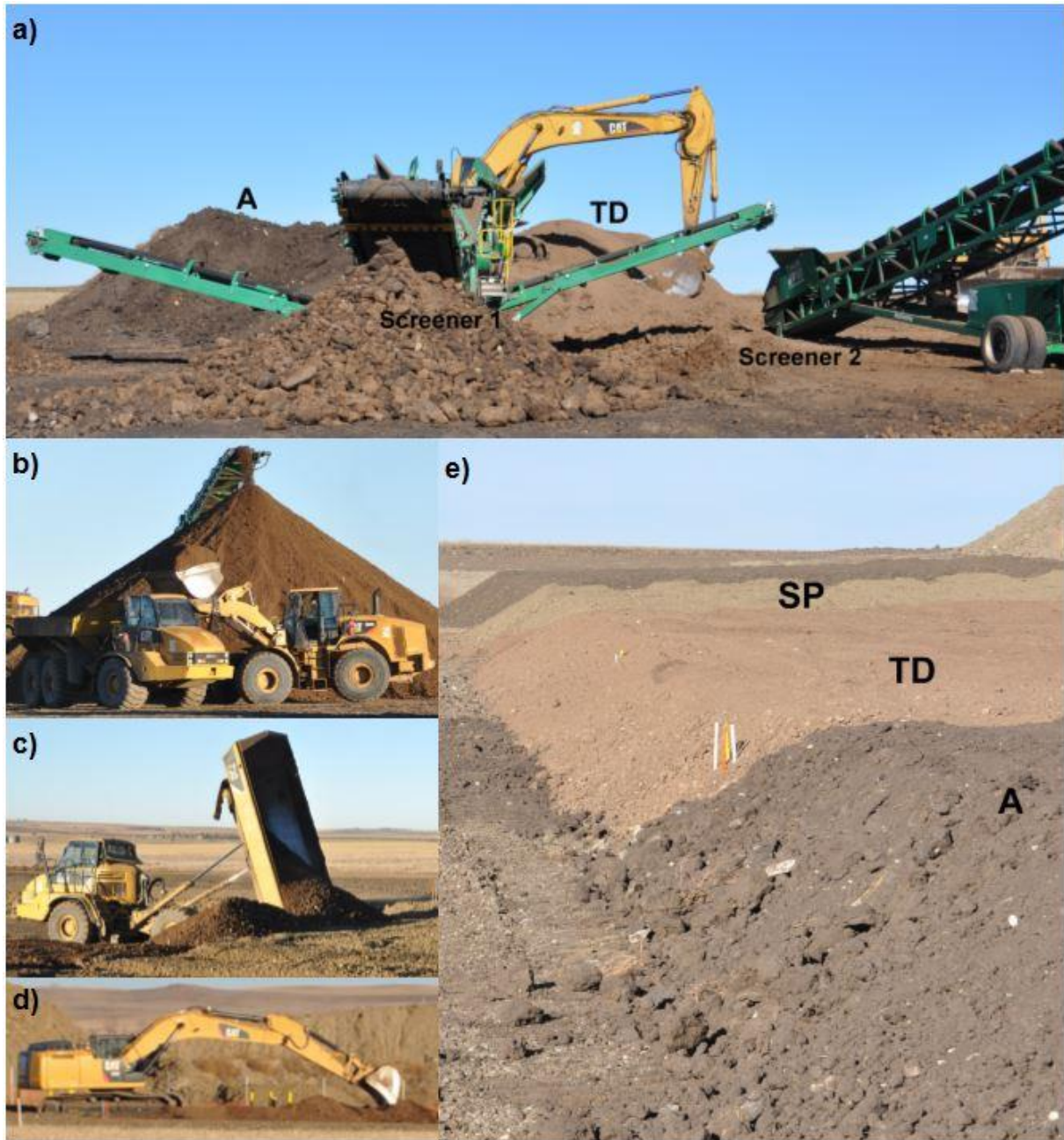
Figure 12. Photographs showing the soil mixing process. Pane a) shows two different soil materials, A and TD, prepared to be placed in alternating bucketloads to the screeners. Soils were taken from the staging pile (b) via trucks to be dumped into plots (c). Plots were smoothed with an excavator bucket (d). The stark color differences of three plots with different materials (A: native, non-contaminated topsoil; TD: crude oil contaminated subsoil material treated by thermal desorption; SP: crude oil contaminated subsoil material) are shown in pane e). The finalized plots were completely filled and leveled to match topography of the surrounding area.
