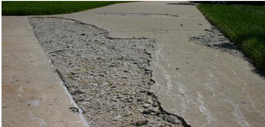
Figure 15. Pavement damage due to freeze-thaw cycles (civildigital.com)
