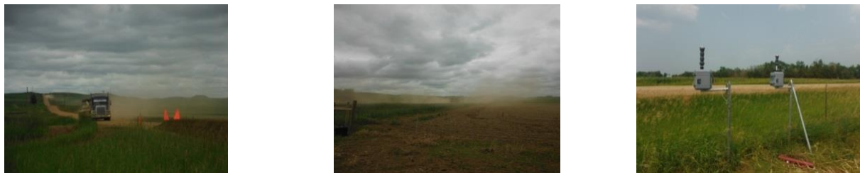
Figure 7. Photographs at Location 1. Construction work at Location 1 (left); Photo of dust generated by one truck at Location ( middle); setting 2 at Location 1 south of the road (right).
