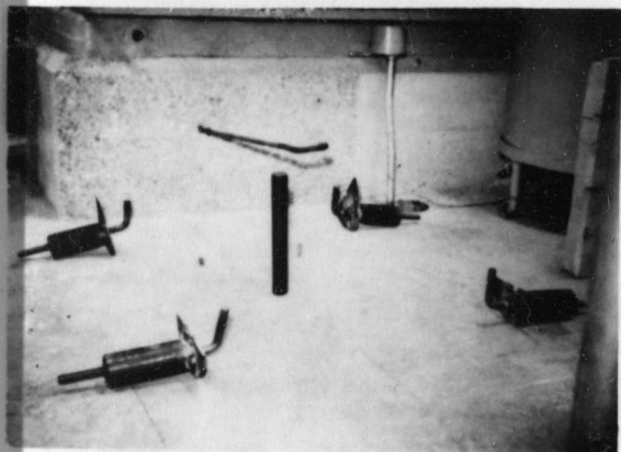
Figure 4-a. Photograph showing the roughed up portion of the engine foundation, the anchor "holds" and the dynamometer hold-down anchor bolts.
