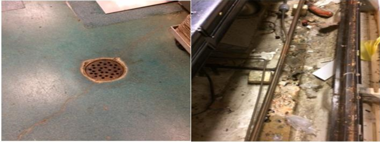
Figure 5. a) Floor drain. b) Soiled interior of display case. Source: Image by David Walpuck
