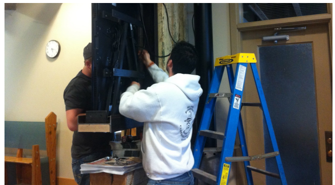
Ty Pritchard, left, and Nick Lippert install TV monitors for the Renaissance Hall dashboard.
