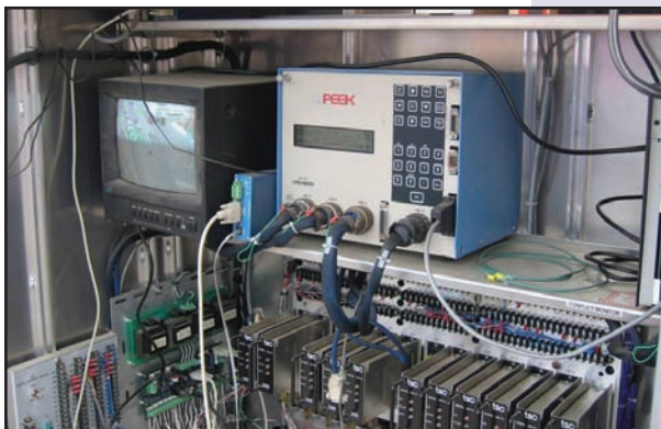
Traffic Signal Control Cabinet (City of Minot)
