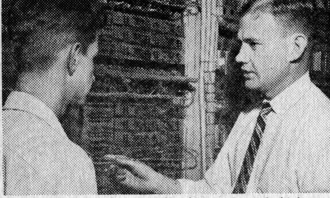
"10:45 a.m. Before any modifications can be made, it's important that I check apparatus and wiring options. That's what I'm doing here at the Remote Control Terminal equipment."
