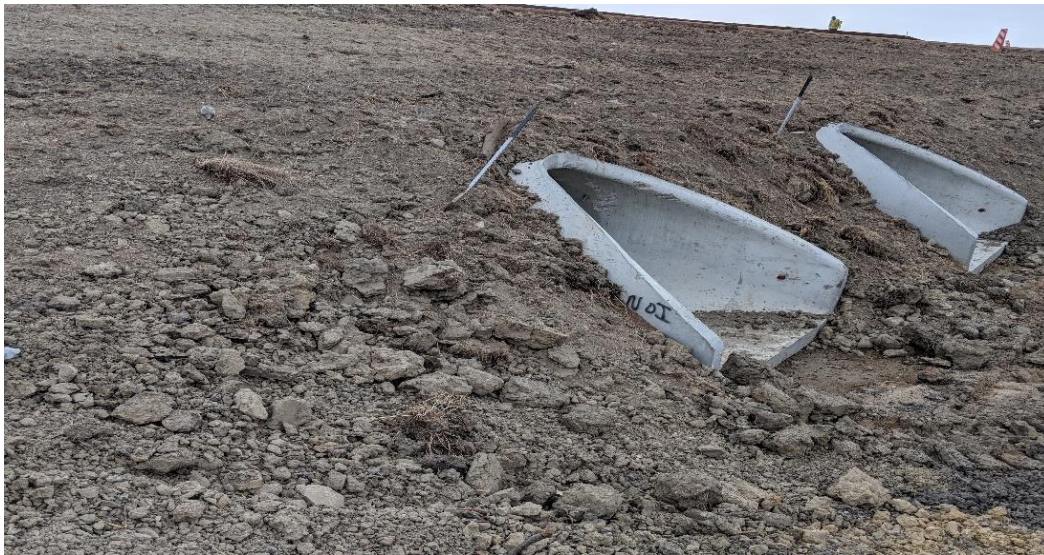
Figure 11: Pipe Work at HWY 1804, North Dakota
