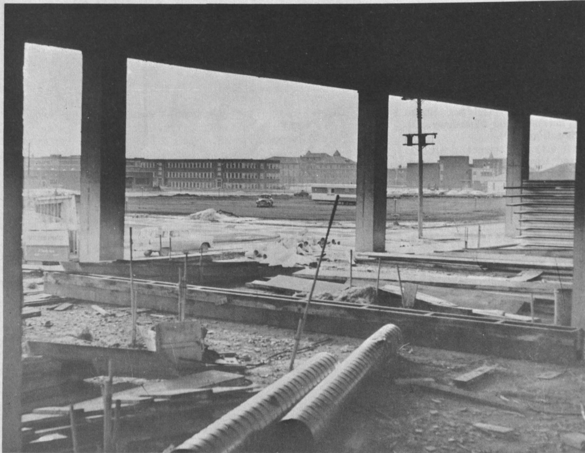
WALSTER HALL , new $750,000 building going up on campus, is still a skeleton. It frames the campus in this view.
