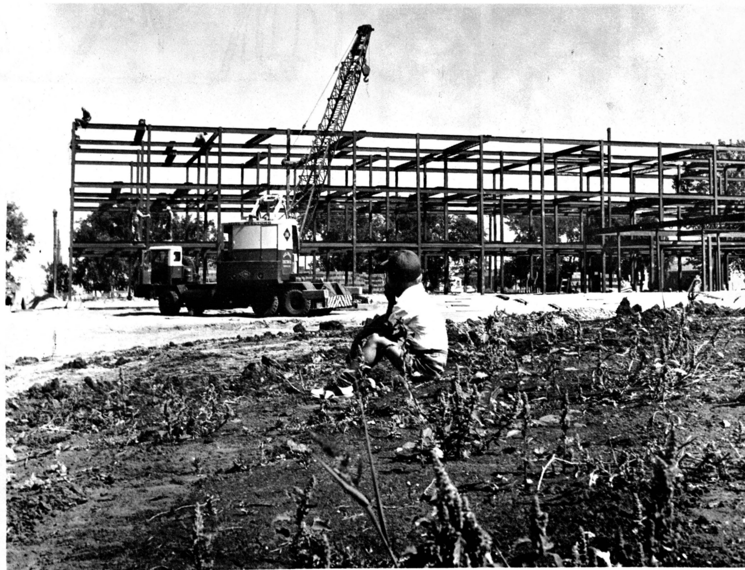
NEW DORMITORY goes up on NDSU campus. It is one of two under construction and will help alleviate the student housing shortage. Several more dormitories will be built in coming years.
