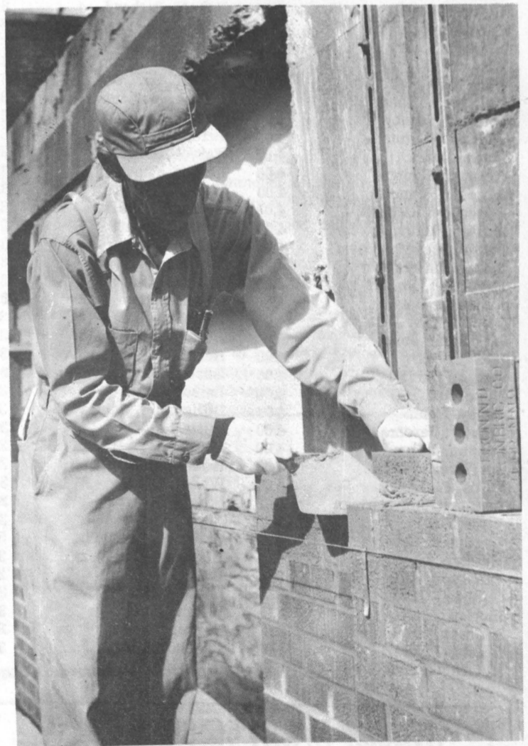
AG ENGINEERING GETS NEW FACE as Joe Prerosil of the Kvamme Construction Company helps lay the bricks.
