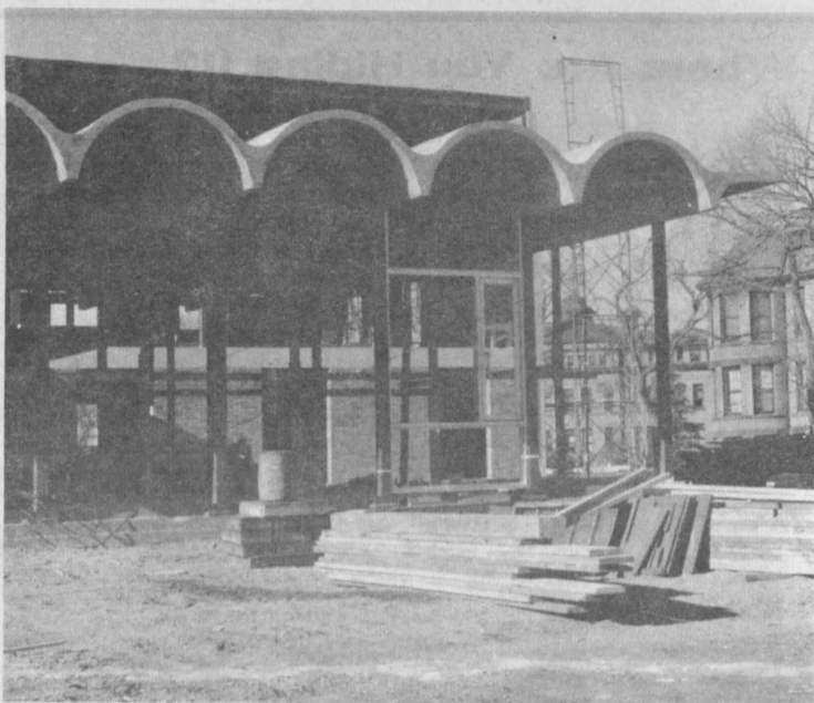
LOUNGE AREA FOR THE WOMEN'S dormitory has a corrugated roof referred to by architects as a "vaulted concrete slab" construction. The wavelike curves of the roof were molded in cardboard forms as a new experiment in vaulted slab construction according to Don Johnson, president of the Fargo firm responsible for the general construction of Burgum Hall. The concrete curving roof will also serve as a ceiling.
