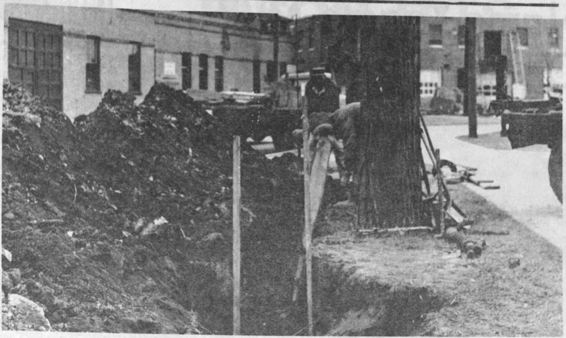
FIRE HYDRANTS for better fire protection are being installed on the NDSU campus. In the mean time the grounds looks quite torn up as is
