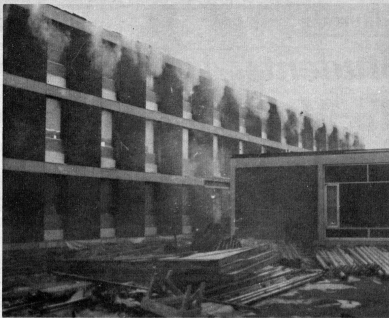
The fire that broke out Friday in the new addition to Reed Hall, men's dormitory (above) resulted in only minor damages. The fire was thought to be caused by sparks from a welding torch.
