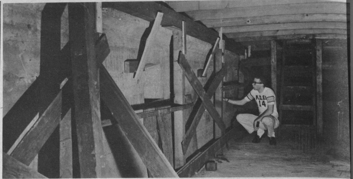
CHECKING THE SWIMMING POOL in the fieldhouse is Lee Grim, AAS-jr. Grim is underneath the floor boards inside the actual structure of the pool.
