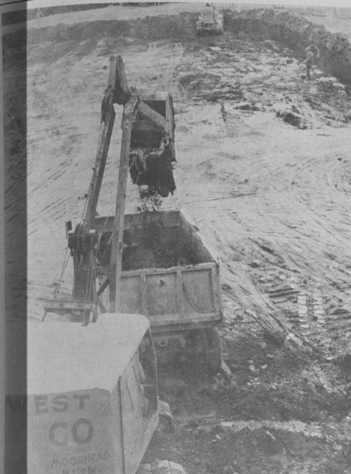
CONSTRUCTION BEGINS on the new women's residence hall being built in conjunction with the North Residence Complex. The hall will be ready for occupancy by fall quarter, 1965.
