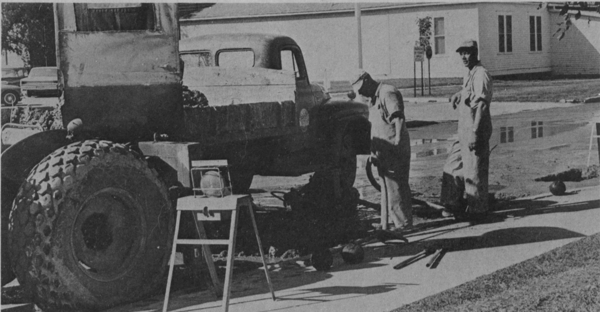
A BROKEN WATER MAIN outside the Union tied up traffic and curtailed the use of water in that building for the better part of last week. Workmen above are pumping mud from around the pipes prior to repairing them.
