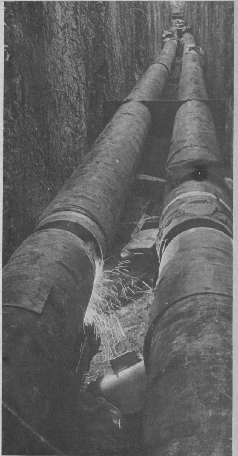
STEAM PIPES being laid between the campus power plant and the new nine-story dorms are welded together.
