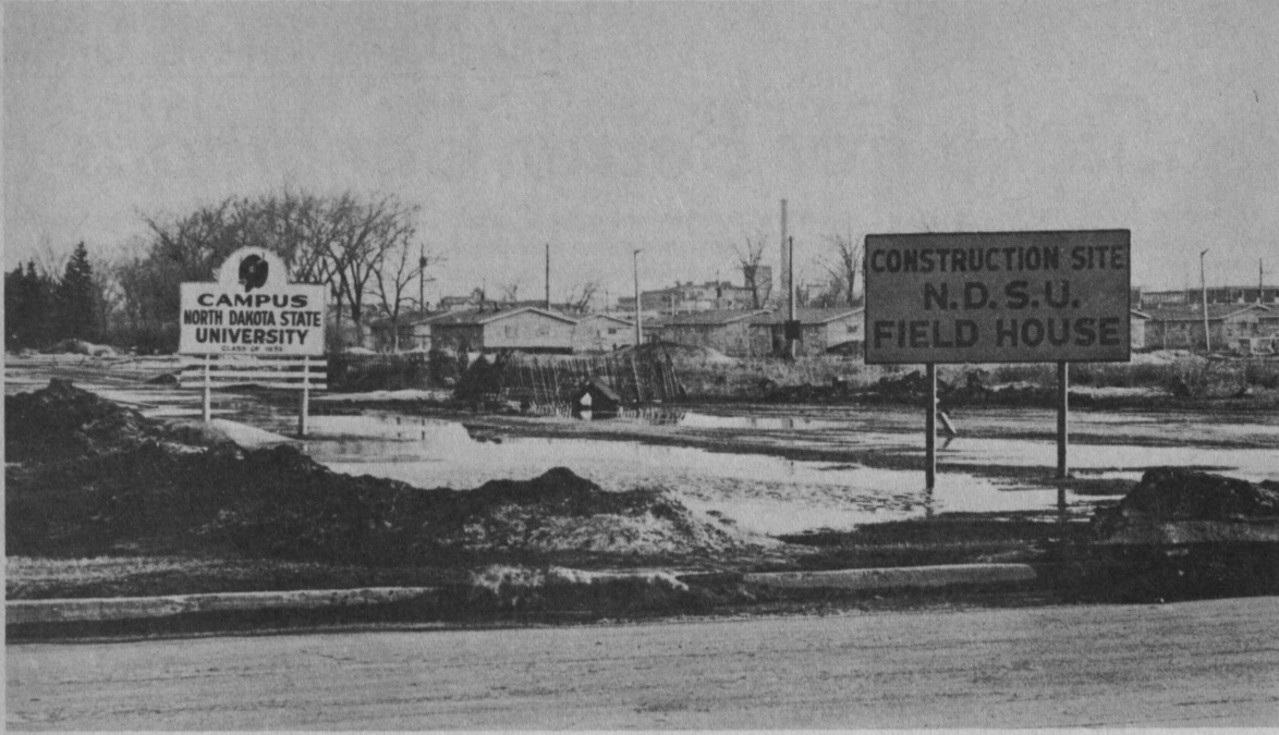
Snow and water cover the construction site of the $2.9 million Physical Education Building, just east of the stadium. Specifications call for a tartan covered main floor, an oval track, swimming pool, handball court, wrestling area and gymnastics room to be housed in the three level plant. (Photo by Loberg)
