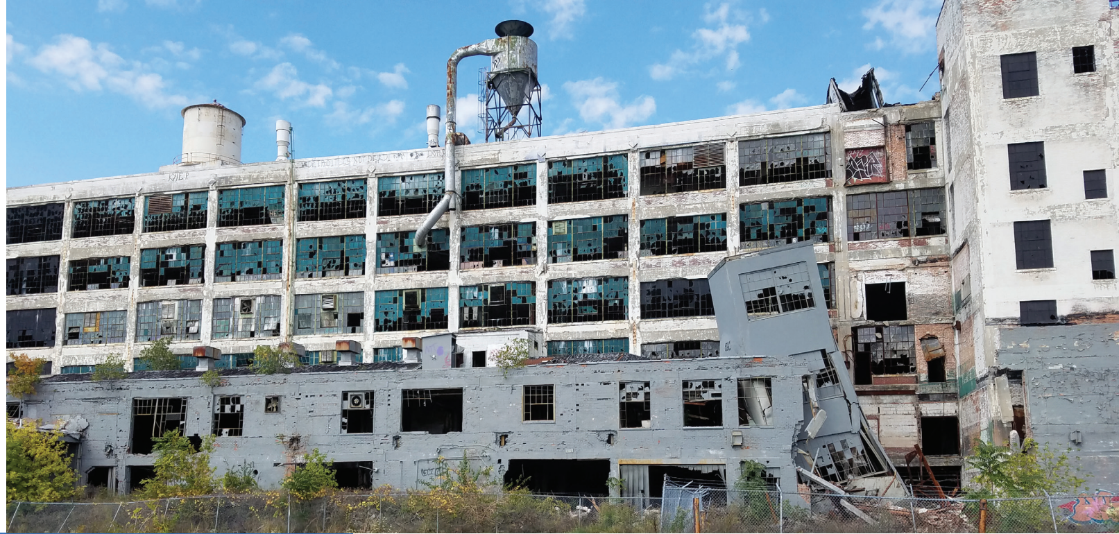
Deteriorating and collapsing loading area and vegetation on south side of building.
