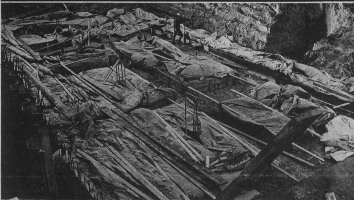
A lone workman, upper center, adjusts the foundation forms being constructed for the new addition to the power plant. When completed sometime next spring, the addition will house the gas-fired boilers that will replace the present coal fed ones.
