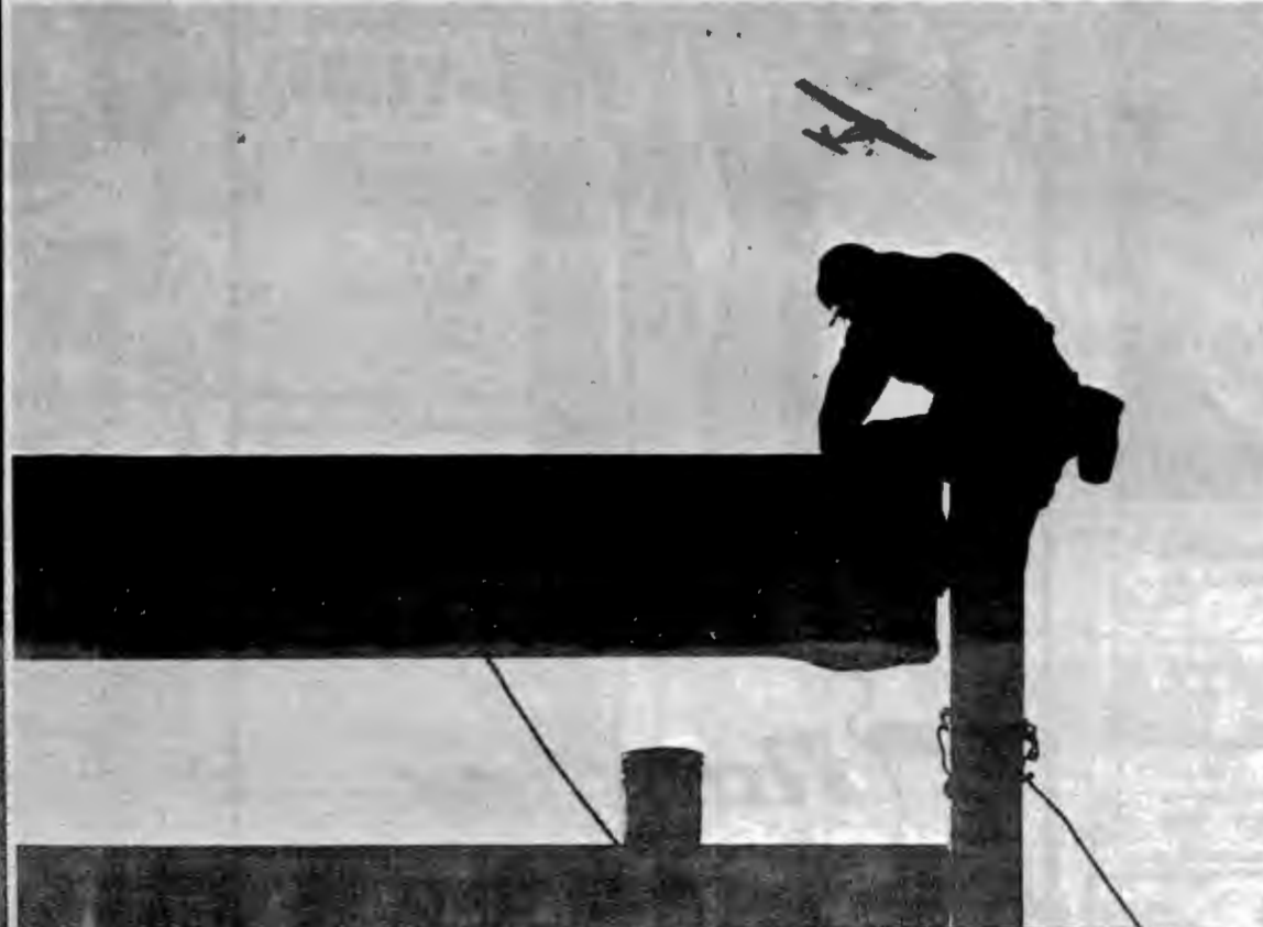
A small airplane appears about ready to knock a worker from his precarious perch. The construction job is the new addition to the heating plant replacing the present coal-fired boilers.
