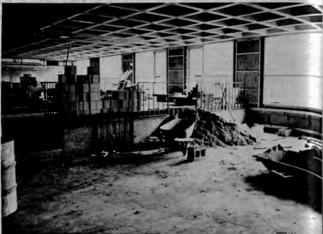
Work continues on the construction of the new high-rise dormitory. That structure, along with the new dining center, are scheduled for completion this fall.
