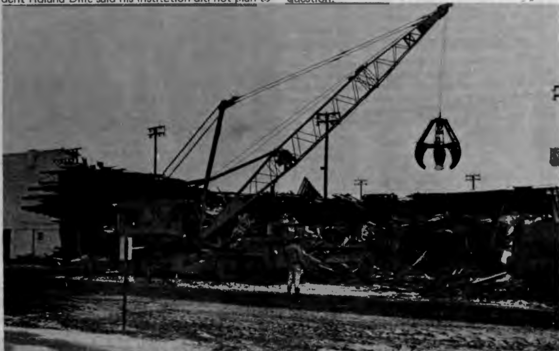
Destruction of the present south stands in Dacotah Stadium is more than half complete last Saturday. The facility is scheduled to be replaced by new seating designed to accommodate more than twice as many fans. The new stands, whose construction is slated to be complete by mid July, will cost about $150,000.
