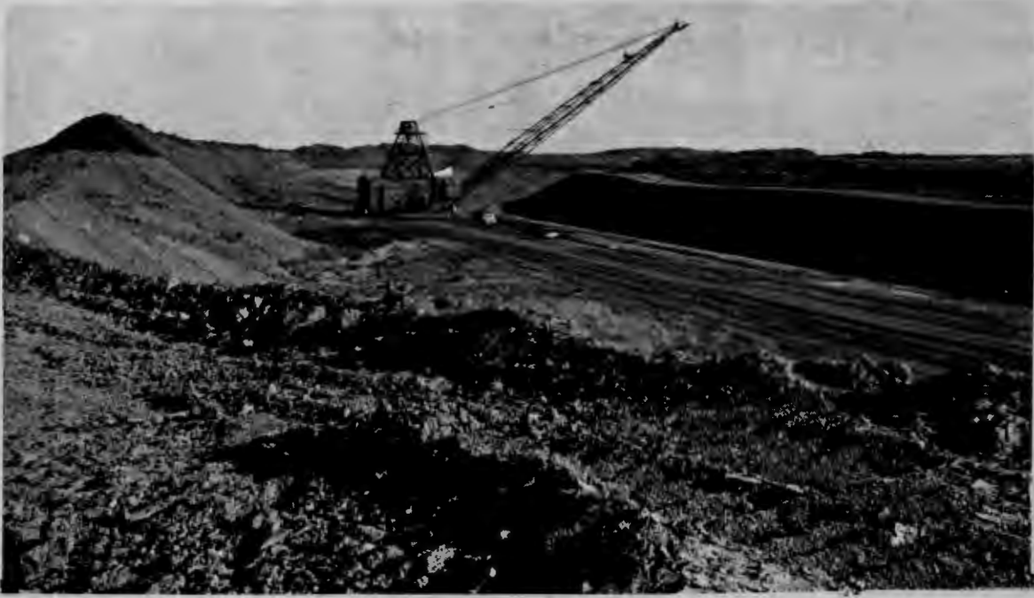
Digging goes on at the McClusky canal, part of the Garrison Diversion project.
