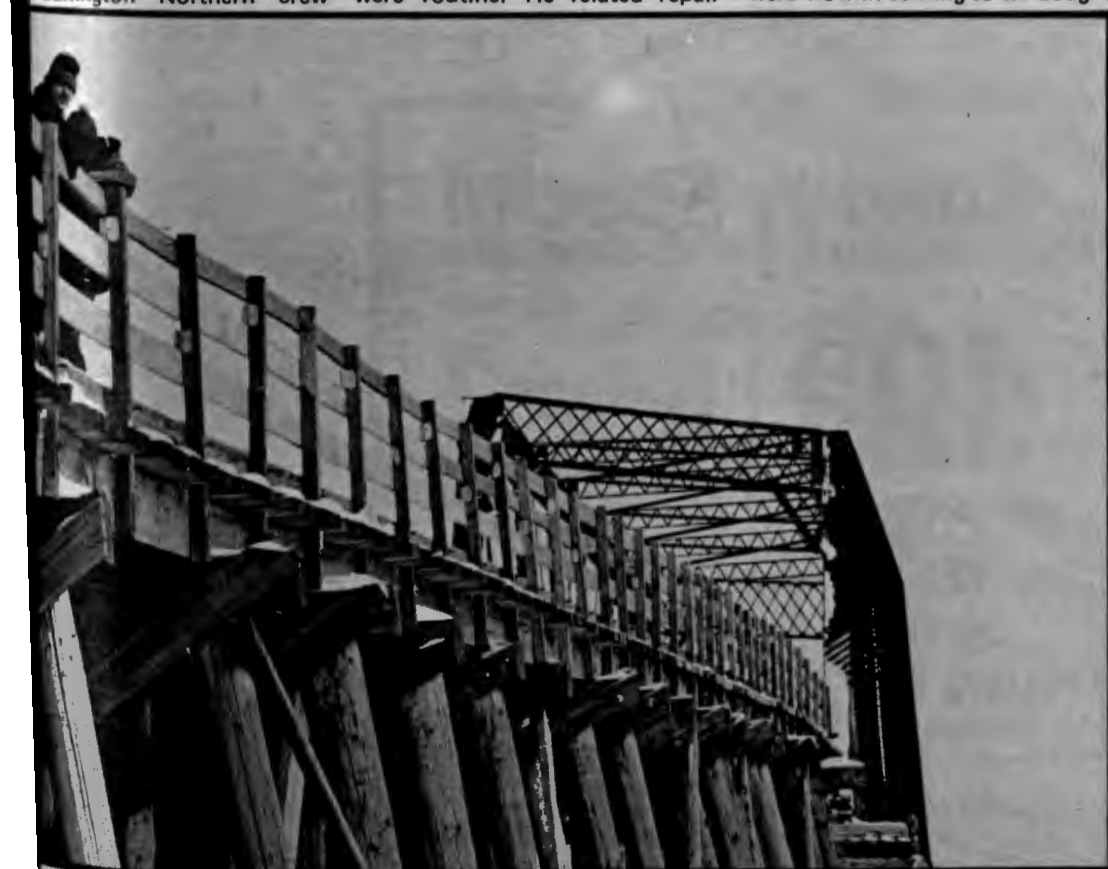
12th Avenue Bridge is back!!!!!! It is now possible to get from campus to I-29 and West Acres without going through Greater Metropolitan Fargo. Burlington Northern repair crews finished their work yesterday afternoon. (Photo by Gary Grinaker)
